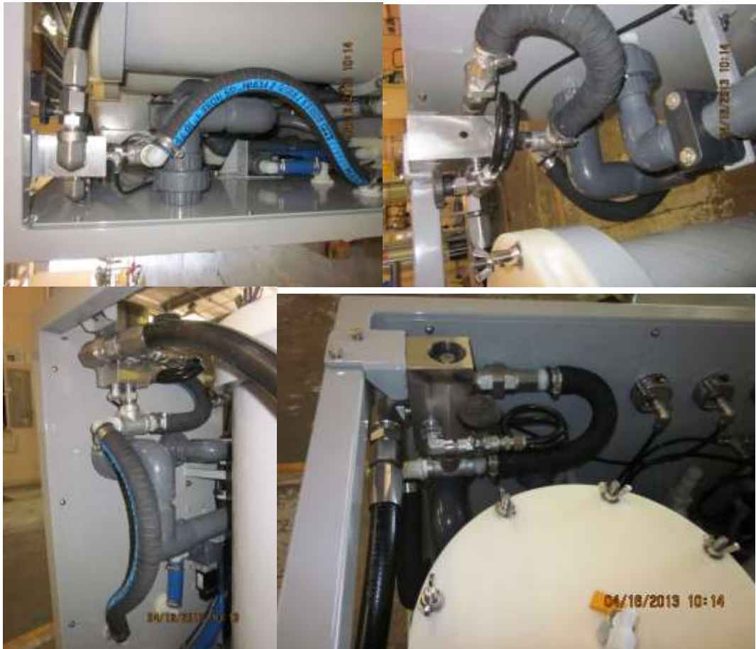
Installation for the new valve 60-4663
